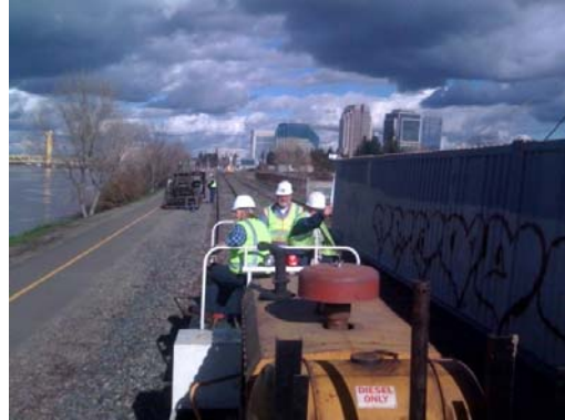
Janet, Frank, and Jack riding out on the MOW work train. to place rail anchors.
