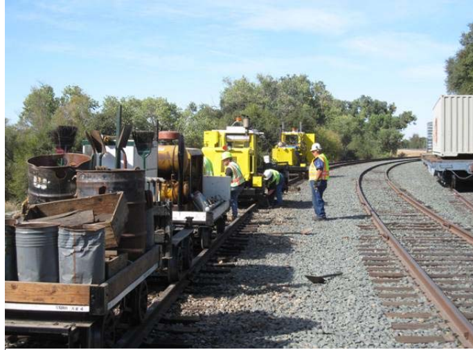
Saturday lineup of MOW equipment changing out ties along the SSRR mainline at Baths.
