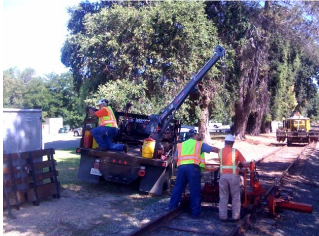
Chris and Mike place the section gang machine on the track to change ties while Harry gets gas in the truck.
