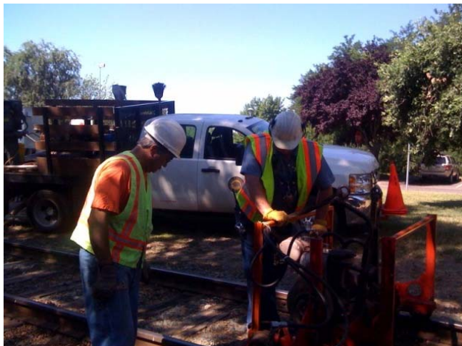
Chris and John Rexroth working on the section gang machine changing out ties on the SSRR.
