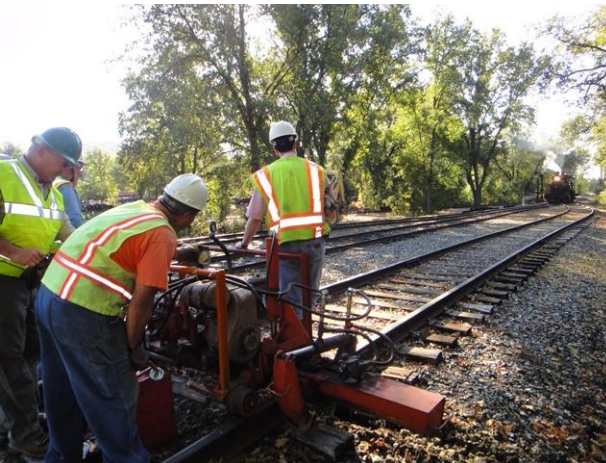
John R. and Rob prepare to fuel the section gang machine while John C. and Frank keep an eye on the Sierra #3 approaching the work area.
