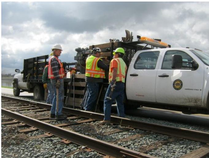
The MOW crew uses the crane on the CT to load and unload the section gang machine as well as change the broken working heads of the machine.
